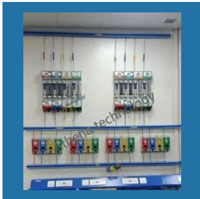
Gas Purification Panel
