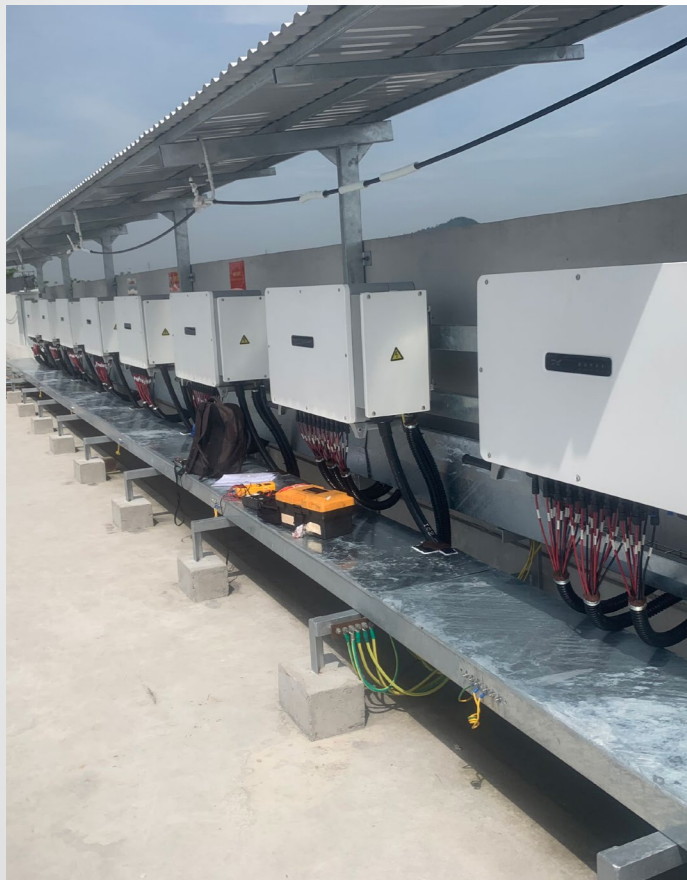
2MW PV Rooftop Project in Vietnam
