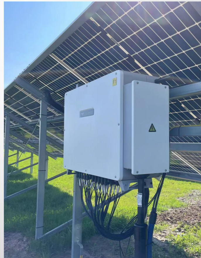
PV Power Plant in Poland
