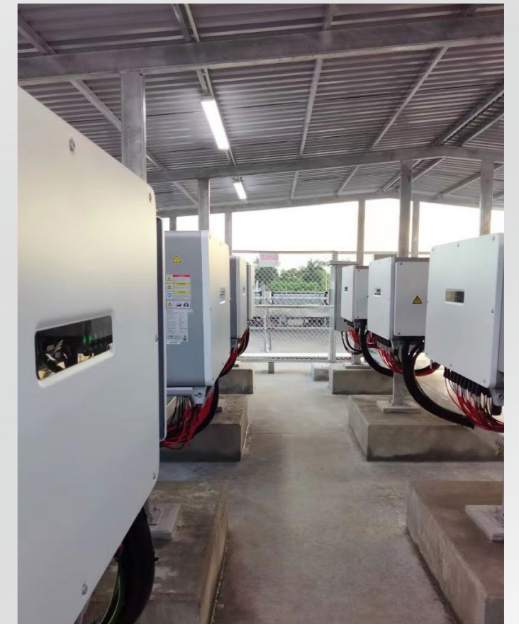
2.5MW PV Rooftop Project in Vietnam
