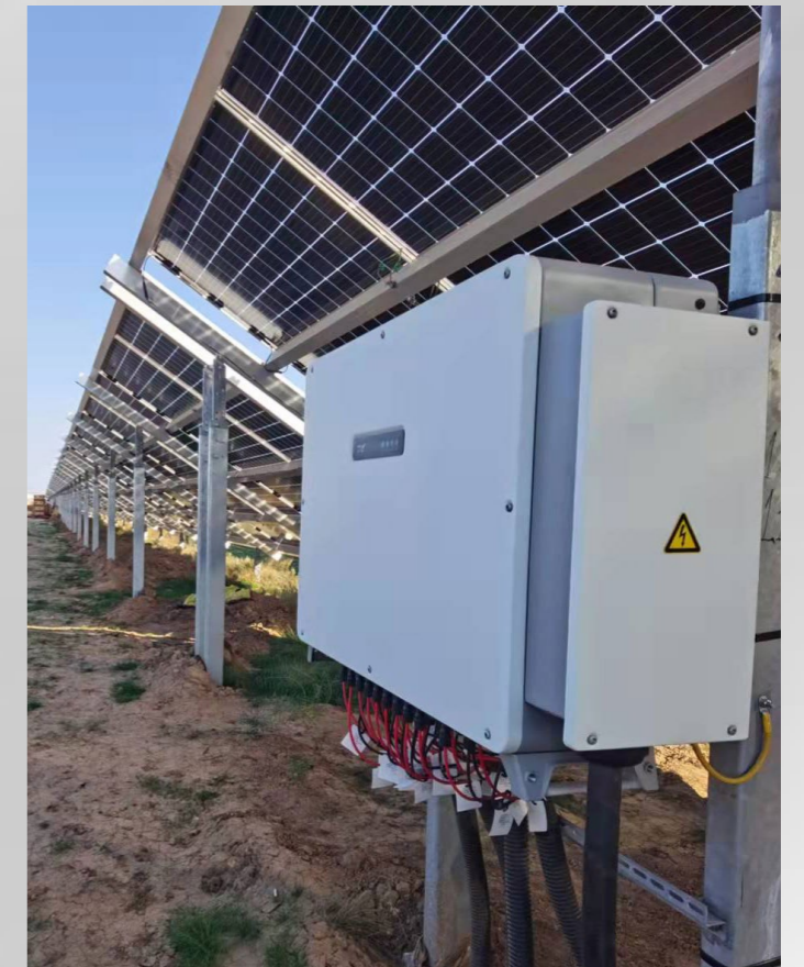
115MW PV Power Plant in Europe
