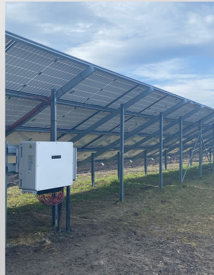
2MW PV Power Plant in Poland
