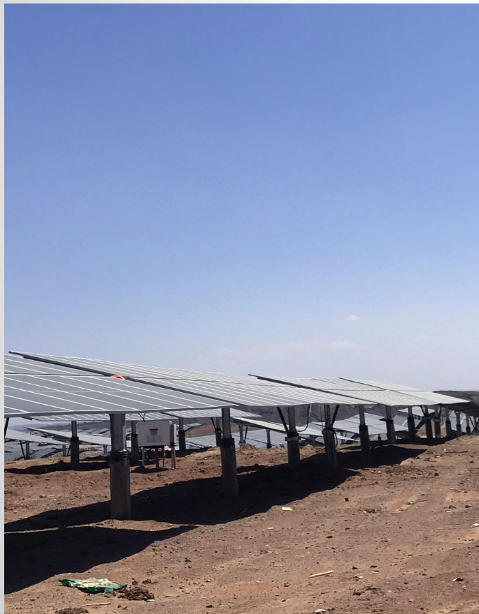
150MW PV Power Plant in China
