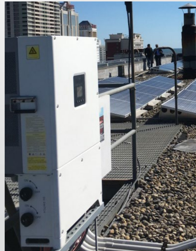
Atlantic County Government Office Rooftop System in New Jersey, USA
