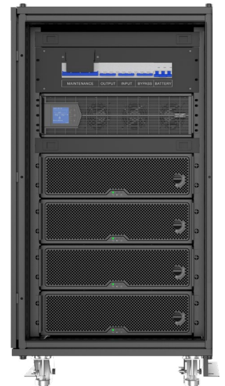
100Ah lithium-ion =battery system cabinet
